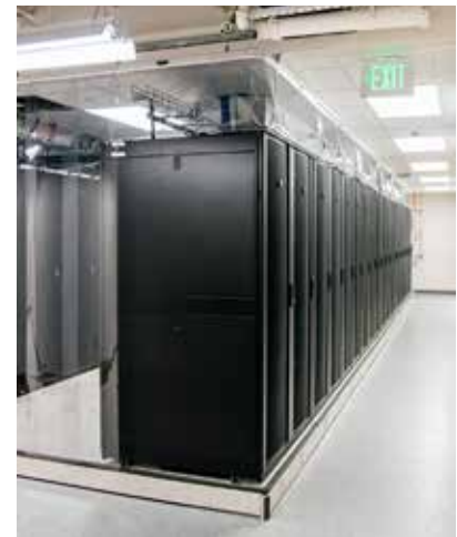
Overhead cable trays are easily used with DIS' Isolated Platform.
