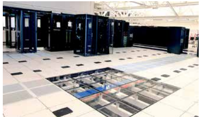
Isolated floor system installed at UC Berkeley.
