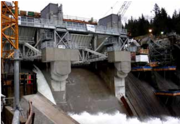
Critical equipment at the Ruskin Dam is protected with a 3D isolation system from DIS.
