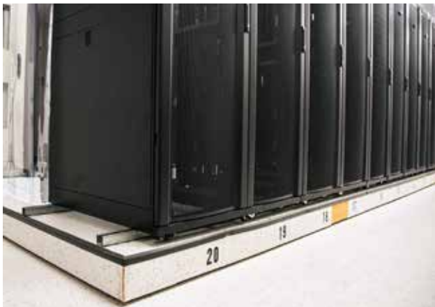
40' long Isolated Platform houses two banks of servers and IT equipment.
