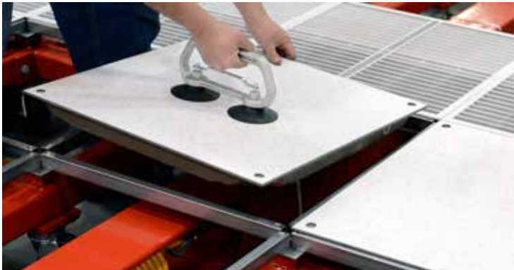
The platforms use standard size computer floor tiles.
