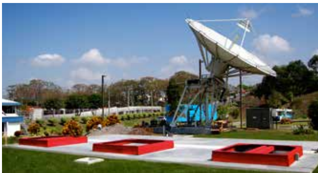
A modular isolation system ready to accept a modular data center.
