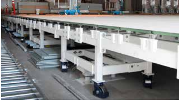
Installation of a 16,000 square foot isolated floor at the UC Berkeley Computational Research and Theory Facility.
